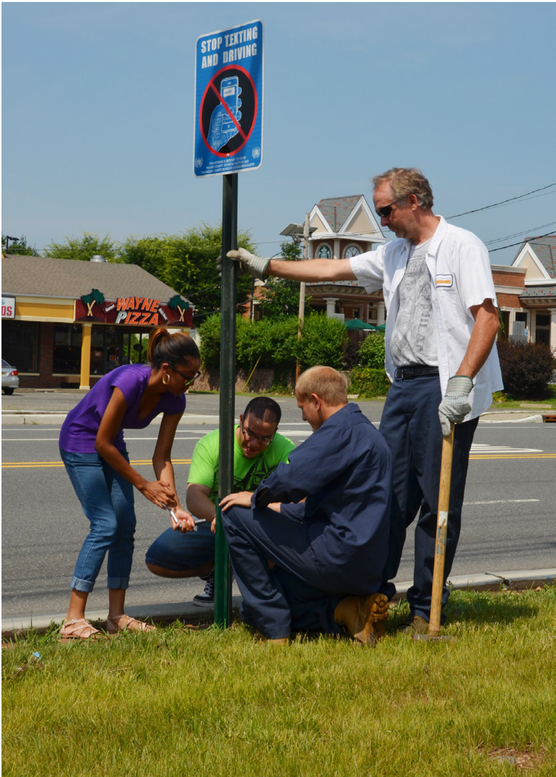
Photo Caption: PCTI graduates Devin Broughton (Clifton) and Anthony Gonzalez (Paterson) assist in installing the “Reject the Text” sign on Hamburg Turnpike in Wayne with members of the Passaic County Engineering Department.
